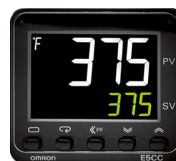
Electronic Controller located on door
